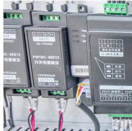
Containerized energy storage , Microgreen.ca
