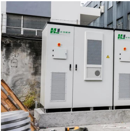
Port of spain energy storage container
