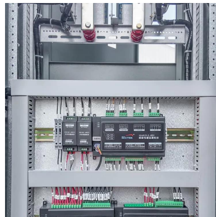
Huawei Luna the storage system
