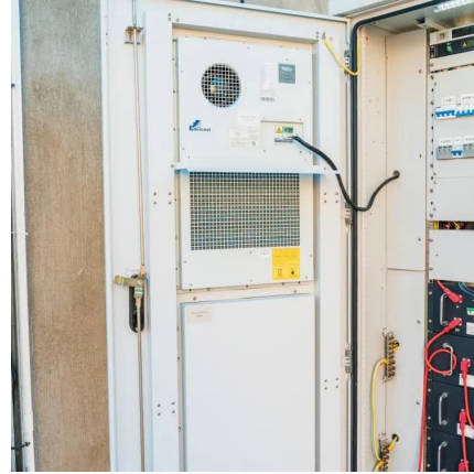
Energy storage container, BESS container
