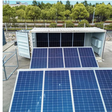
20-foot energy storage container
