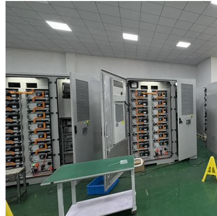
Mobile solar container , PV power, energy , Power MOVEit.tech
