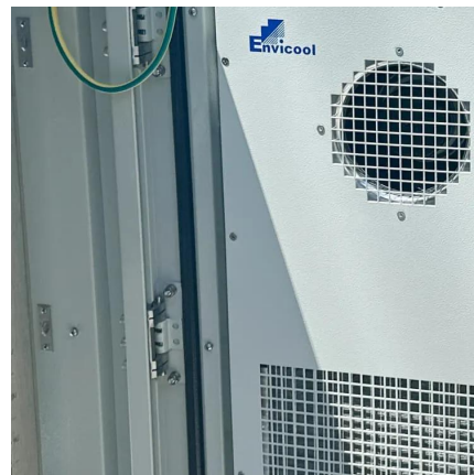
Lithium-Ion Battery Charging Safety Cabinet
