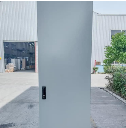
Battery cabinet.Lithium battery storage ...
