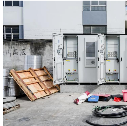
Energy storage container, BESS container
