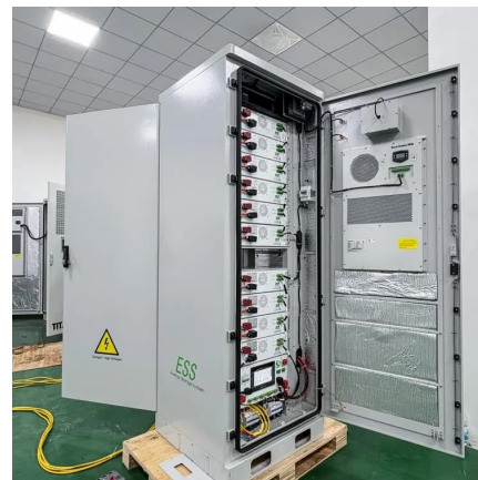
Off grid container power systems -- Off-Grid Installer
