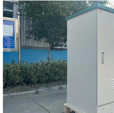
containerized battery storage , SUNTON ...
